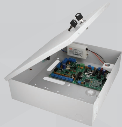
COMFORT CM9001 Controller in secure cabinet
