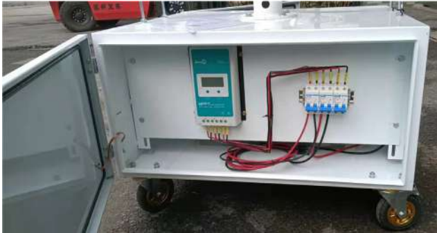
Controller + Surge protector + Breaker
